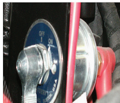
Internal battery disconnect
